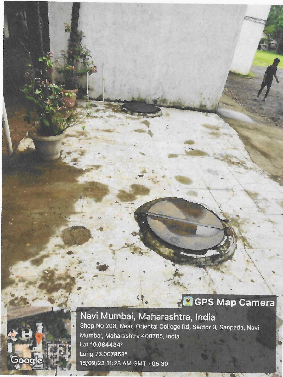
Water Storage tank for Fire Safety
